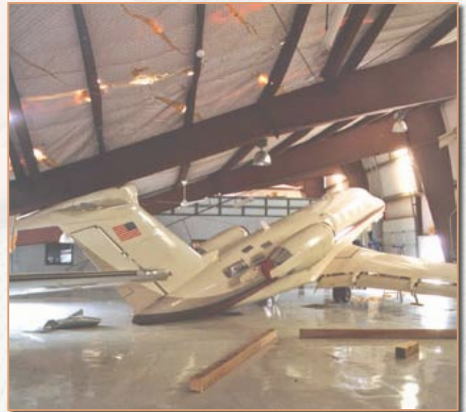
Rigid frames in failed corporate jet hanger
