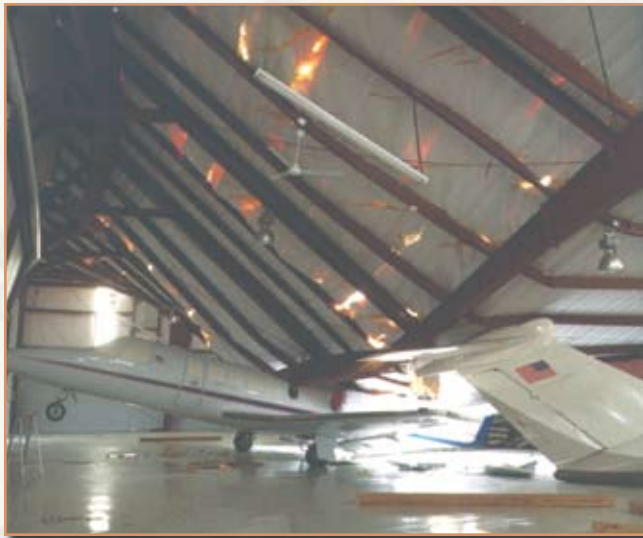
Failed corporate jet hanger
