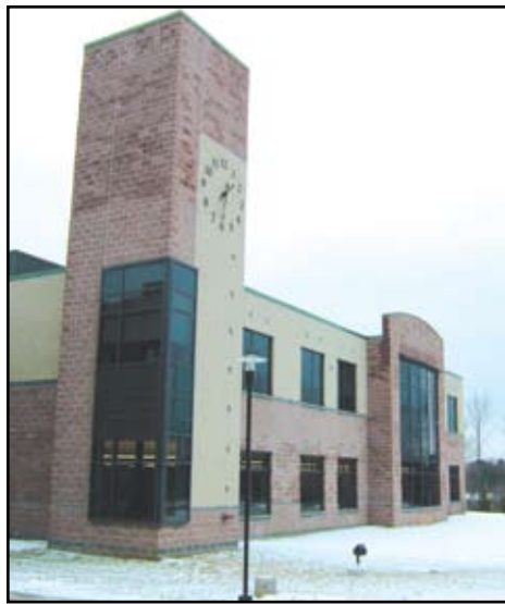
The walls of this school have architectural CMU veneer over loadbearing CMU.
