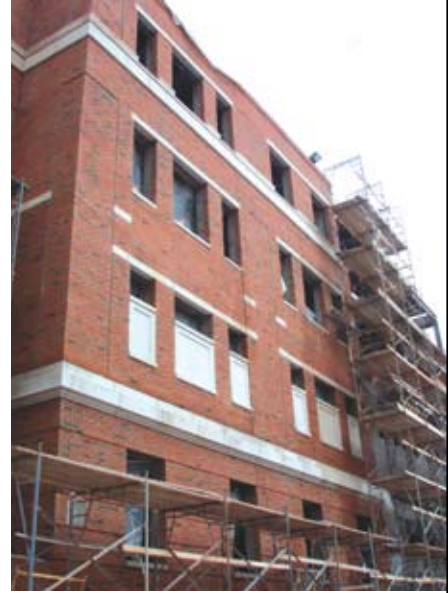
For this university building, the walls are brick veneer with reinforced CMU. The CMU acts as shear walls for the steel frame.
