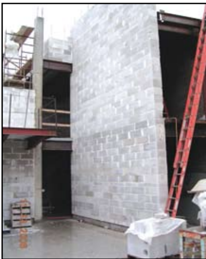
Loadbearing walls constructed of autoclaved aerated concrete (AAC) masonry units for a church addition.
