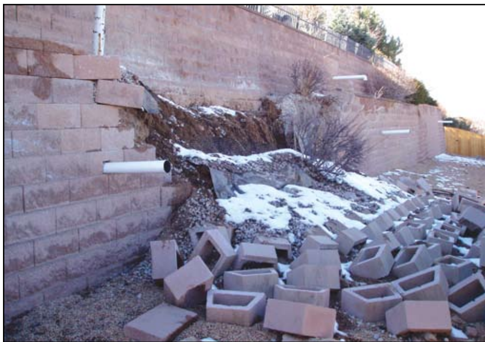
Figure 4: Geotechnical / structural interaction failure of retaining wall
