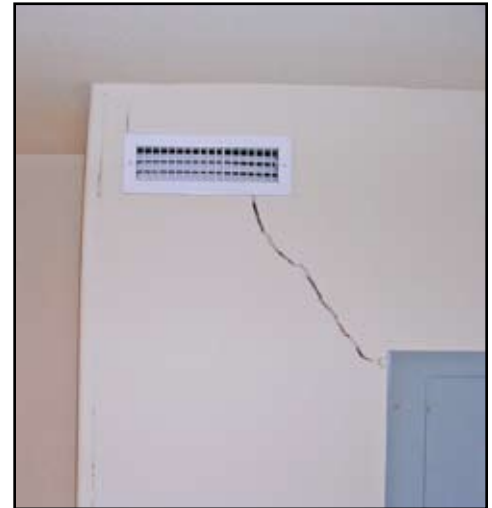
Figure 7: Significant drywall distress resulting from undesirable soil and structure interaction
