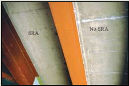
Figure 4: Effectiveness of mix design using SRA to control the cracking in bridge decks
