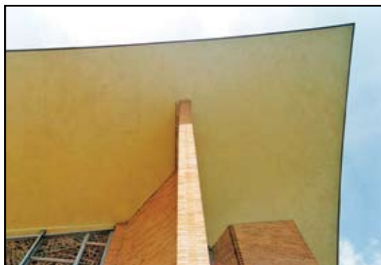
Figure 2: Top of original fin wall shows bowing of wall and displacement at canopy soffit.
