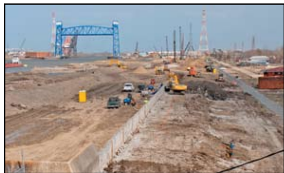
New Orleans, LA, 2-12-06 -- 9th Ward, U.S. Army Corps of Engineers remove dirt from the failed 9th Ward Levee in preparation to remove the old Sheet Piling and replace it with Cat 4 Sheet Piling and reinforcement "H" Piling. Courtesy Marvin Nauman/FEMA.
