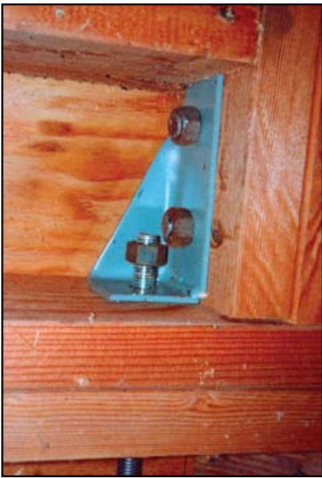
Solid sawn wood can experience shrinkage exceeding 3/4 inch per floor. This photo shows shrinkage nine years after installation.
