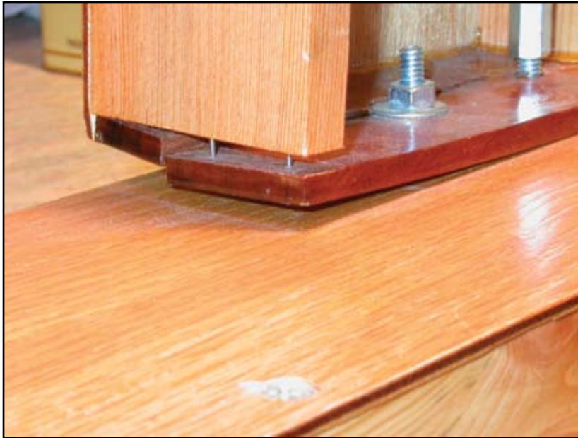
Loose holddown connections allow shear panels to lift. The result is cross grain mudsill failure as shown, or nails bending and breaking.
