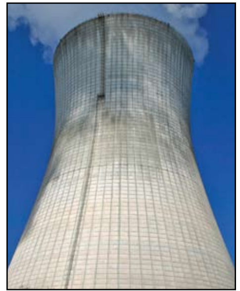
Located at St. John's River Power Plant in Jacksonville, Florida, the Unit No. 2 hyperbolic cooling tower is 450 feet tall and 360 feet in diameter.
