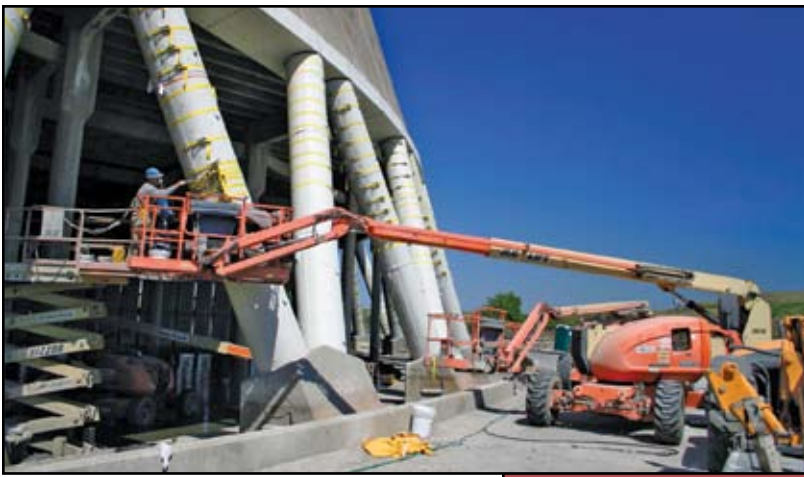
Once the jacket was around the column, the strap was released and the jacket closed around the column. Next, ratchet straps were wrapped around each section of jacket.
