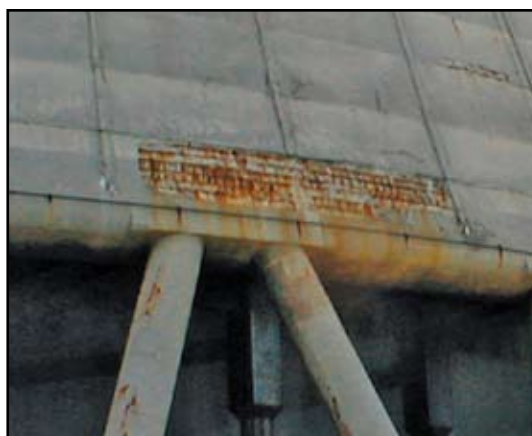
During operation, practically all surfaces in the basin are subject to "immersion" conditions. Columns and lintels are in a "splash zone" environment.
