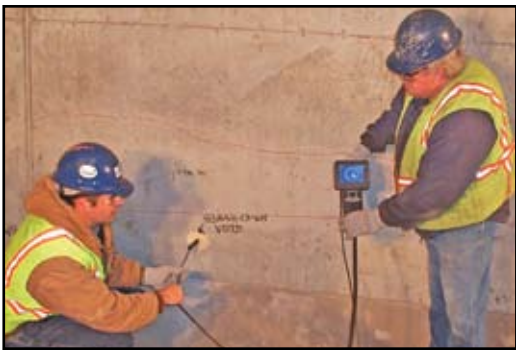
Figure 3: Crew inspecting and recording the condition of the grout and strand using a video borescope
