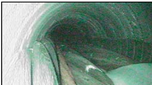
Figure 4a: Example of corrosion – Duct Void
