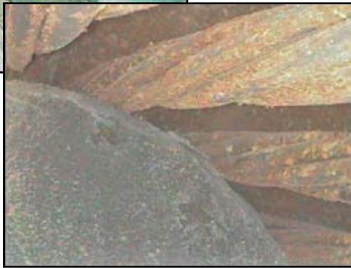
Figure 4b: Example of Level 1–2 Corrosion
