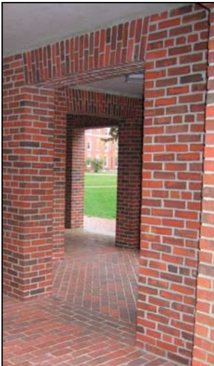
Flat arches known as “Jack Arches” – notice there are no steel lintels. Courtesy of Steven Szycher.
