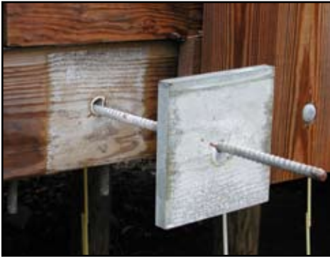
Corrosion of galvanized bridge hardware in contact with alkaline copper quaternary (ACQ) after 3 years of service.
