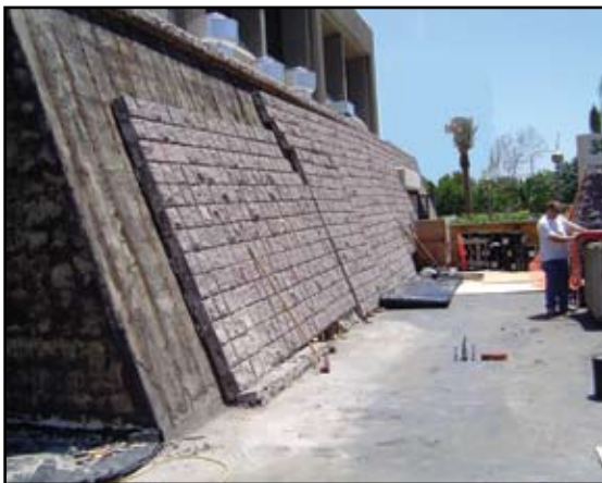
Southwest corner of failed granite wall; south face is sloped 1 horizontal to 3 vertical, while west face is vertical
