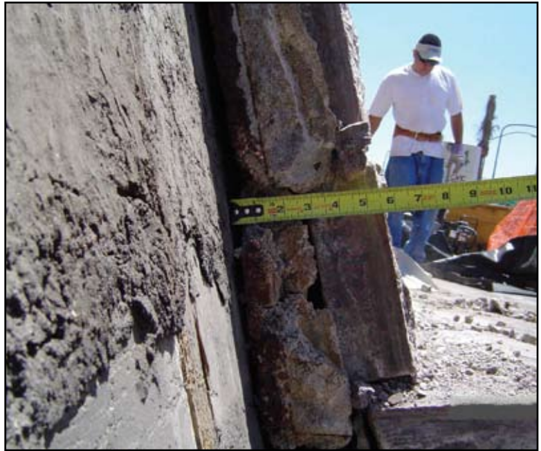
Edge of failed wall where adjacent granite has fallen off
