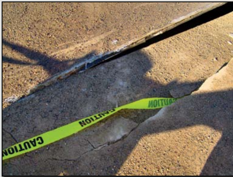
Failed area of deck
