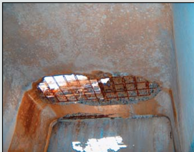
Existing hole in deck
