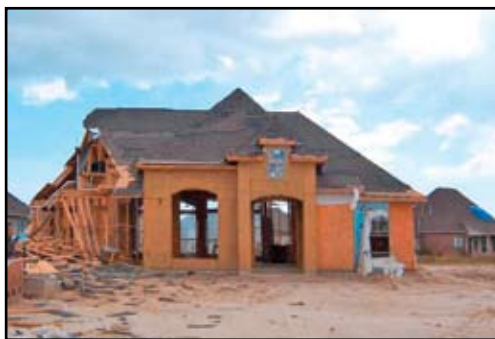
Figure 2: Shear Wall Failure, St. Tammany Parish, LA
