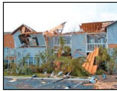
Figure 1: Roof Uplift Failure, Long Beach, MS
