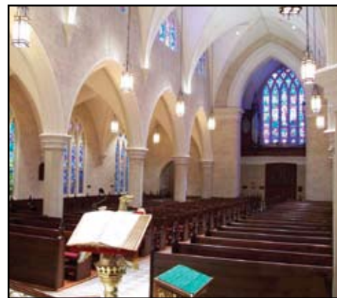
The tower arch at Grace continues to spread and the members bracing the clerestory walls are moving.
