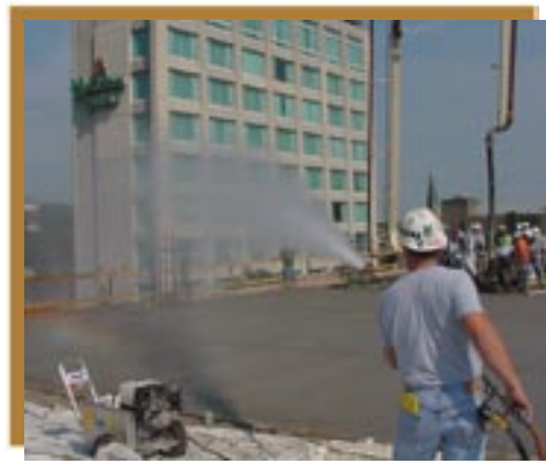
Figure 3: Fogging to increase the humidity of the air above the freshly-cast concrete, and thus reduce the evaporation rate. (Photo Source—K. Hover)
