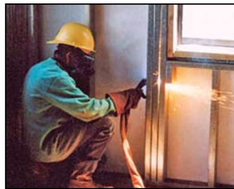
Figure 6: Field Modification of Cold-Formed Steel Structural Framing
