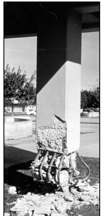
One of four damaged reinforced concrete columns along the east end of the Imperial County Services Building. Imperial Valley, California Earthquake, October 15, 1979. Photo courtesy of USGS photographic archive.
