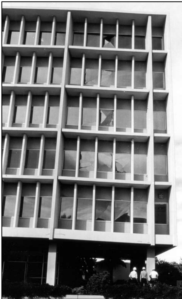
Imperial Valley, California Earthquake, October 15, 1979. East end of Imperial County Services Building showing a row of columns that failed during the main shock. Photo by C. Rojahn, courtesy of USGS photographic archive
