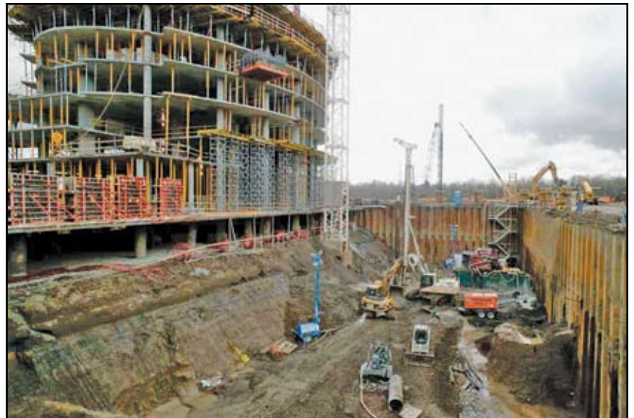
Figure 2: The conventional excavations portion of the site was used to facilitate up-down excavation under the tower. (Photo by Pete Eckert)
