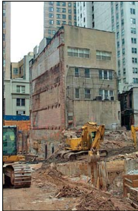
Figure 1: Excessive settlement of this building during underpinning prompted an order to vacate this building, and emergency stabilization measures.
