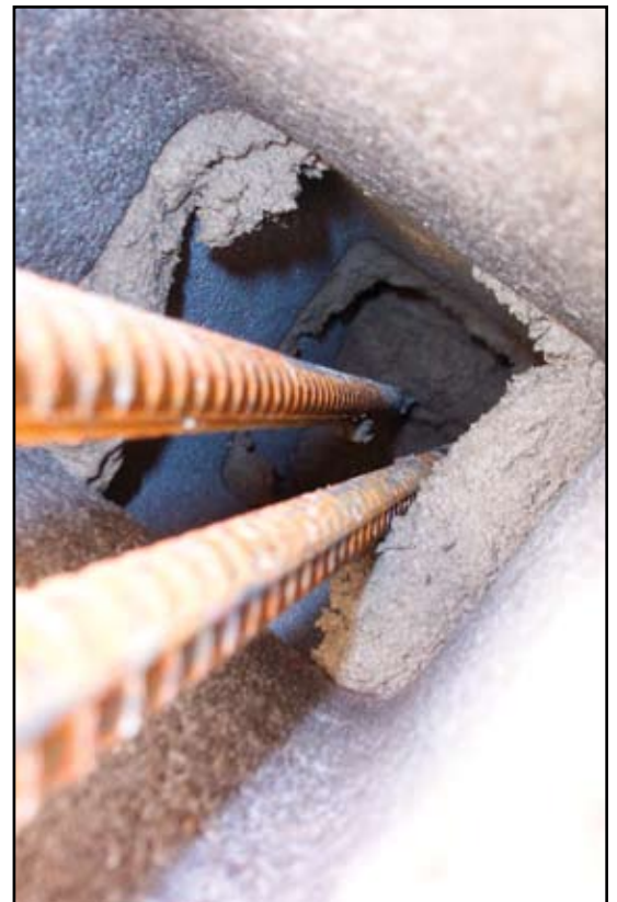
Mortar Extending into CMU Cell.
