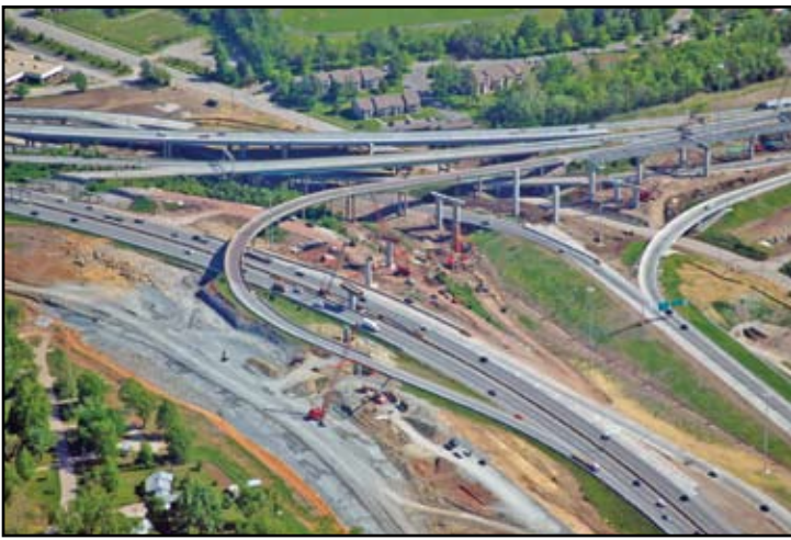
Figure 2: MoDOT mandates that bridge construction at the interchange site not interfere with current traffic flow
