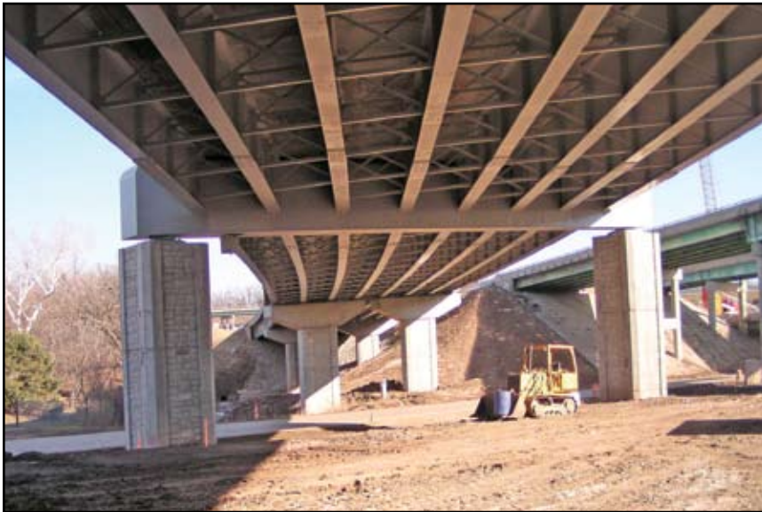
Figure 4: The steel girders welded to the capbeams are continuous and handle torsional moments
