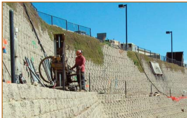
Figure 7: Stiffening of the supporting soils for the lower tier of this retaining wall was accomplished by carefully-controlled and closely-spaced compaction grout injection. Grouting in this case was performed in preparation for a series of tieback anchors that were installed once grouting was complete.
