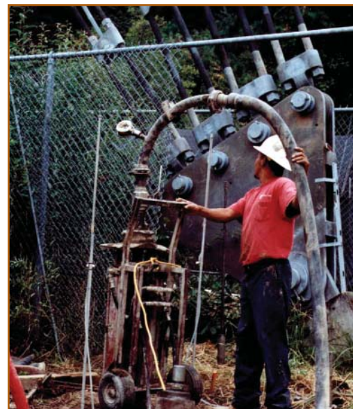
Figure 6: Grout injection being performed at one of the three anchor stanchions for a television broadcast tower.
