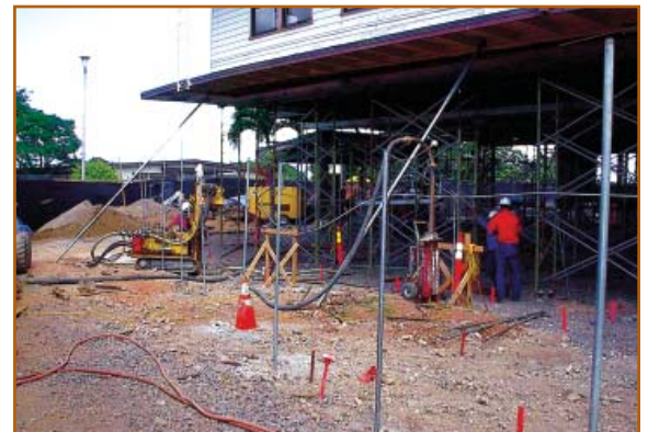
Figure 3: Compaction grouting of an historic military barracks building in Hawaii at the edge of a dormant volcanic crater. The building was lifted off of the ground to provide construction access for various trades, but not a prerequisite for compaction grouting.
