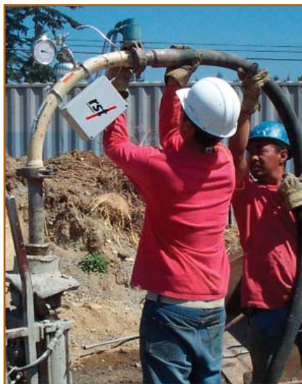
Figure 9: Computer technology is becoming more common in the grouting industry. The manifold shown above contains a pressure transducer and wireless transmitter that works in conjunction with an in-line flow meter. This configuration allows real-time monitoring of pressure and flow for very stiff (zero-slump) grout mixtures.
