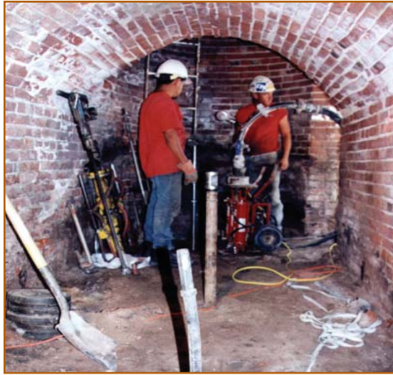
Figure 4: Grout injection for liquefaction mitigation beneath a smokestack at San Diego, California's historic Hotel del Coronado. Such limited-access project constraints are common in the compaction grouting industry.
