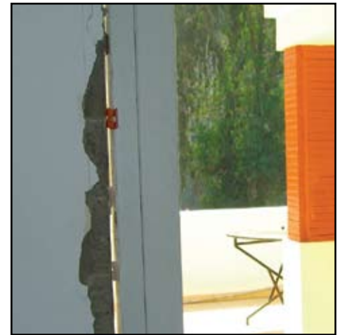
Rotary percussion drilled holes located too close to the masonry surface, causing extensive spalling around perimeter of blast-resistant door.
