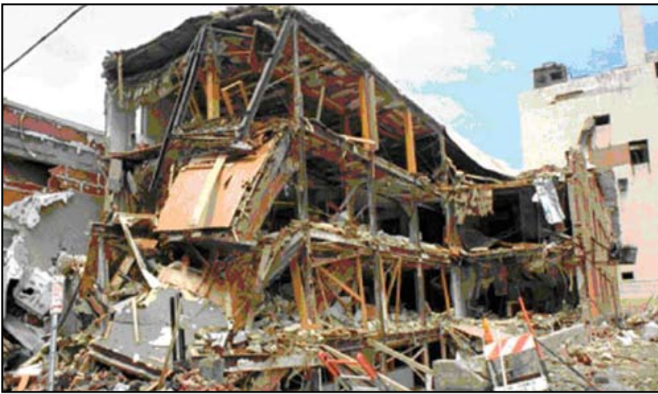
Figure 2: Disproportionate collapse – Oklahoma 1995.
