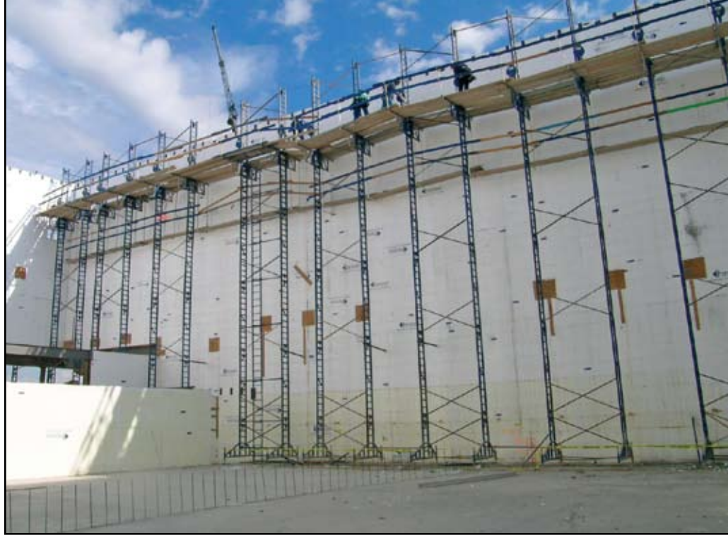
Example of tall wall ICF construction - Megaplex 20 movie theater in South Jordan, Utah.
