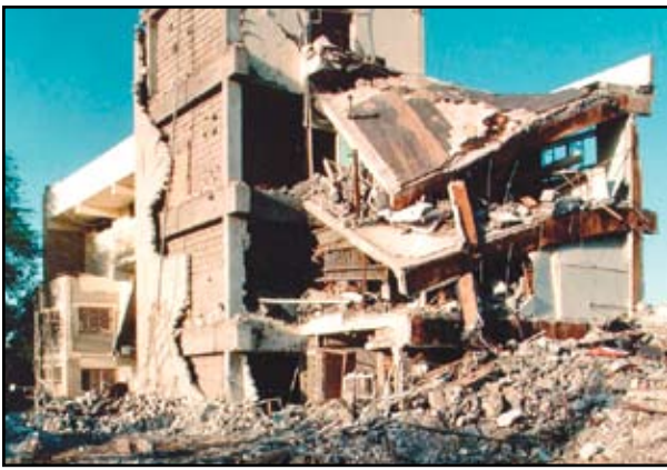
Damage to masonry buildings
