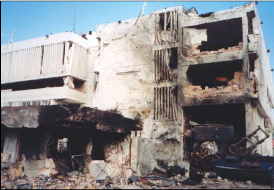
Damage to masonry buildings
