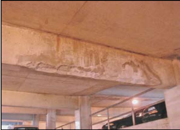
Especially in demanding regions like those near marine environments, garage decking is susceptible to problems related to the corrosion of reinforcement
