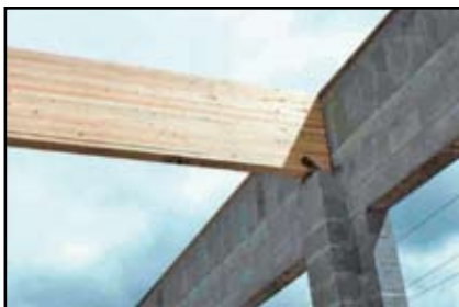
Figure 1: Reinforced glulam used in a roof beam of a commercial building
