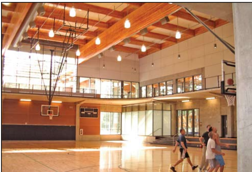
Reinforced glulam girders at WWU main gymnasium. Courtesy of KPFF Consulting Engineers.
