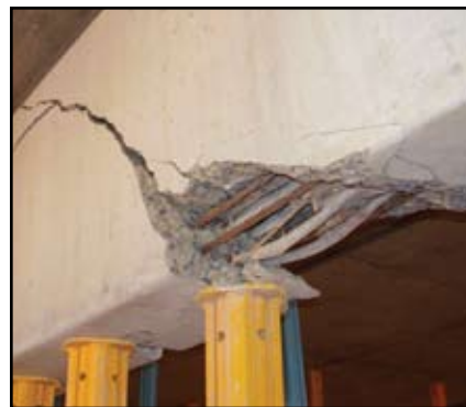
Failed PT beam due to snow overload.
