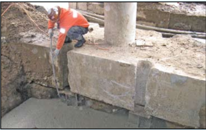
Figure 6: Self-consolidating concrete cast throughout the excavation to top of footing. Slab-on-grade cast back with reinforcement to resist a lateral load of 10% of the expected maximum column load.
