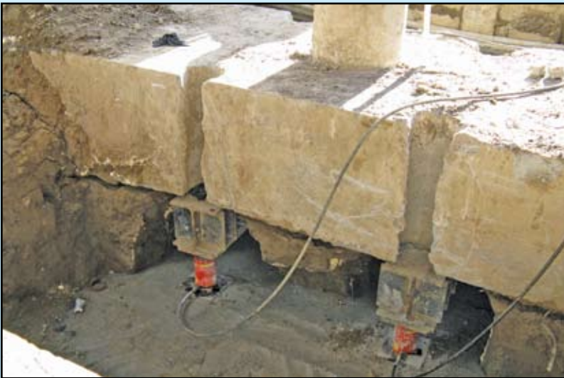
Figure 4: Concrete placed to top of pile cap. Actuators are connected to the same hydraulic pump to ensure the lifting load is distributed to the footing equally.
