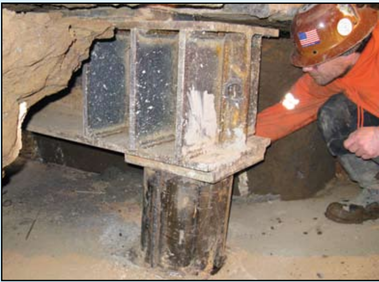
Figure 5: Hydraulic actuators encased in structural steel pipe. Pipe is permanent support for the HP 14 spreader beam and footing.
