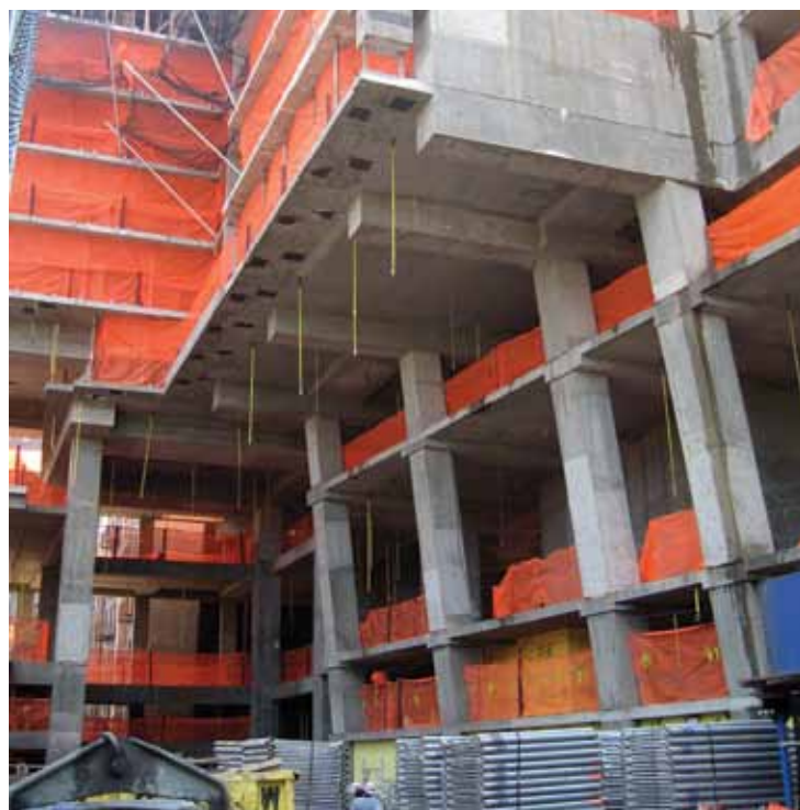
Figure 2: Sloping columns and cantilever beams under construction (prior to the installation of exterior steel frames and the façade system).
