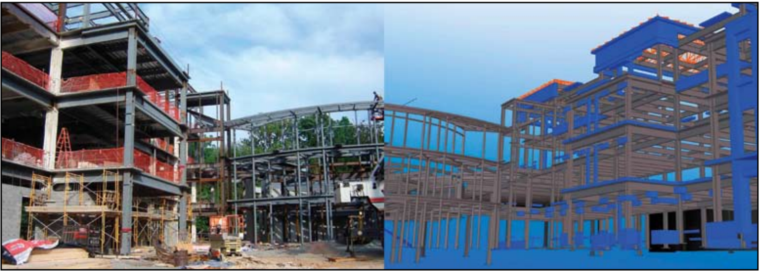
The complexity of the steel-frame building's façade represented a unique challenge, but BIM allowed the project's participants to coordinate any changes in tandem.
