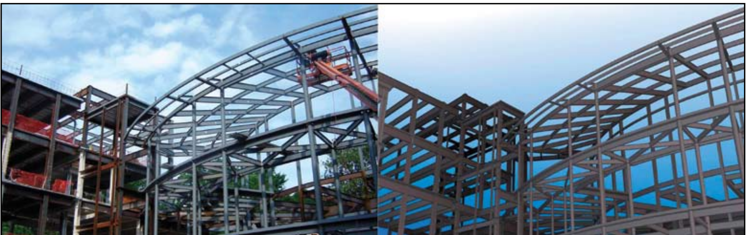
The South Lawn project includes a steel frame building with a masonry and architectural precast concrete skin. Here, the building's steel frame rises over the South Lawn.
