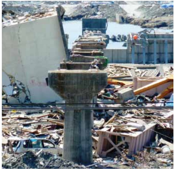
Figure 6: Multiple span and pier failures of a railway overpass and river bridge in Otsuchi, having braced steel plate girders. Courtesy of Ian Robertson, ASCE.
