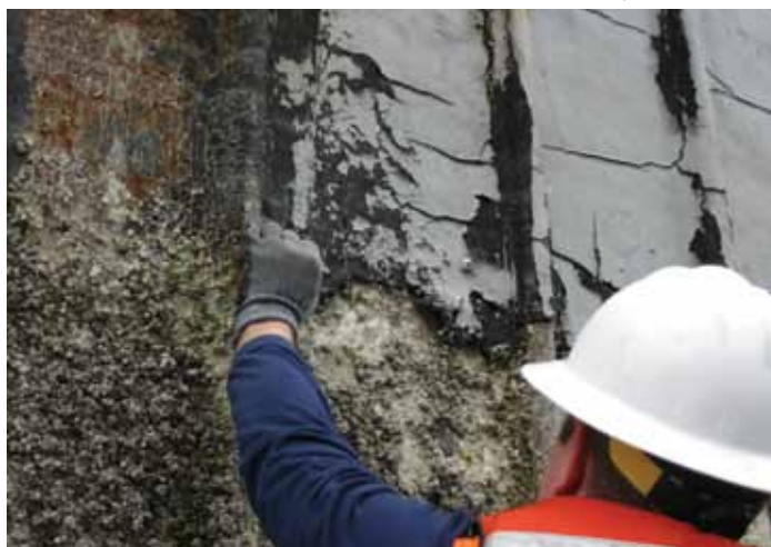
Figure 2: Existing failing cofferdam coating.
