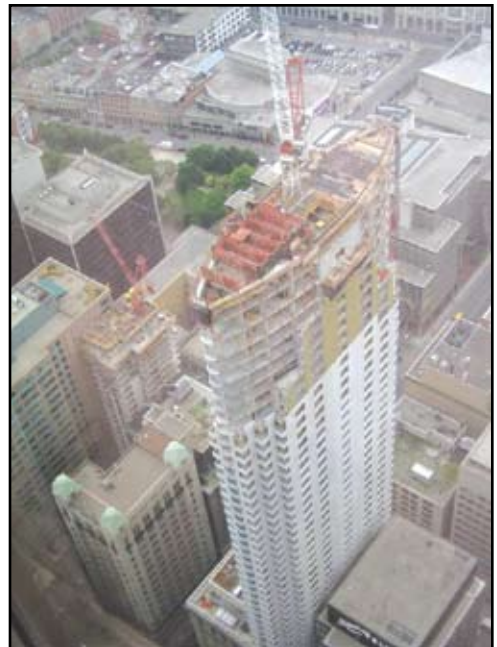
Construction of the liquid tuned dampers at the top of One King West Tower.
