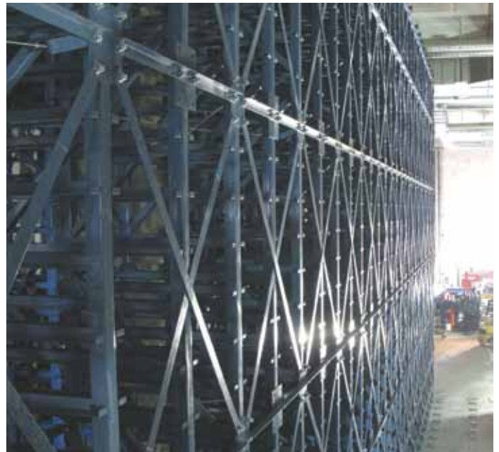
Figure 1: Installation of the high-density automated storage system.
