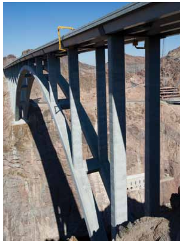
Figure 2: Underbridge inspection trucks work simultaneously on each side of the bridge to facilitate inspection and rope access work. Courtesy of HDR, photographer Keith Philpott.
