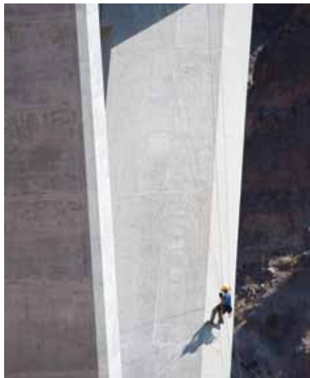
Figure 4: HDR inspector, Al Nelson, inspects the concrete arch rib utilizing a rope-to-rope transfer. Courtesy of HDR, photographer Keith Philpott.
