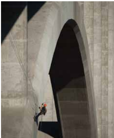
Figure 3: HDR inspector, Craig Smart, utilizes industrial rope access techniques following SPRAT guidelines to gain access to the arch rib and spandrel columns that would otherwise be outside of the reach of traditional inspection equipment. Courtesy of HDR, photographer Frank Huster.
