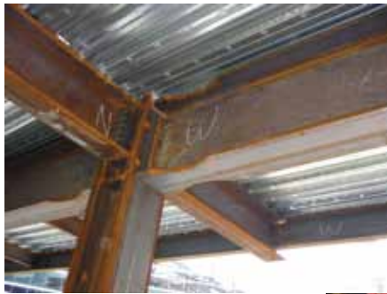
Reduced beam sections (RBS) were selected to meet the Special Moment Frame requirements.
