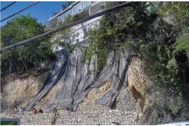
Rare Example of Slope Instability.
