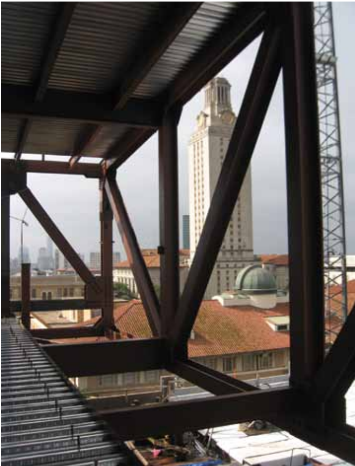
The story-height penthouse trusses cantilever up to 33 feet to overhang the expansion joint.
