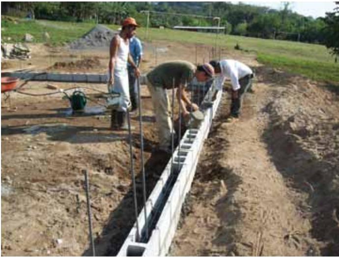
Figure 3: Placing High Slump Concrete for Grout in CMU Cells Near Door Opening.
