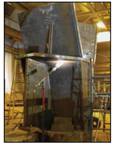
Figure 7: Ground Floor Nodal Connection. Courtesy of Terri Meyer Boake.
