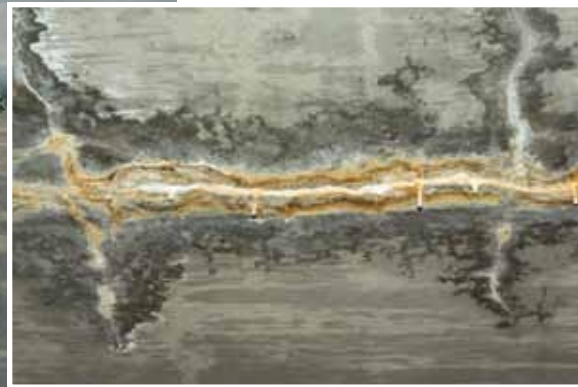
Figure 1: Efflorescence at crack on L1 slab soffit.
