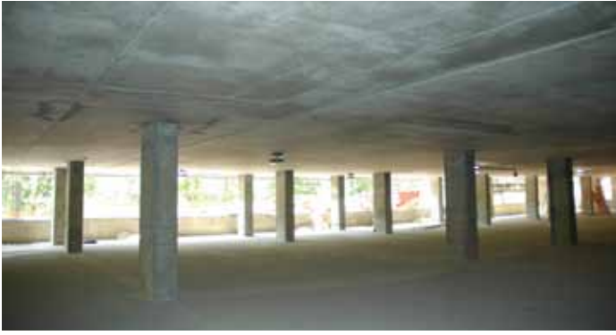
Soffit of First Level slab (standing on slab-on-ground) looking northwest. The first supported level is the most susceptible to RTS cracking.
