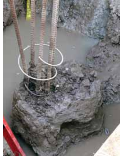
Figure 4: Pile with Settled Grout.
