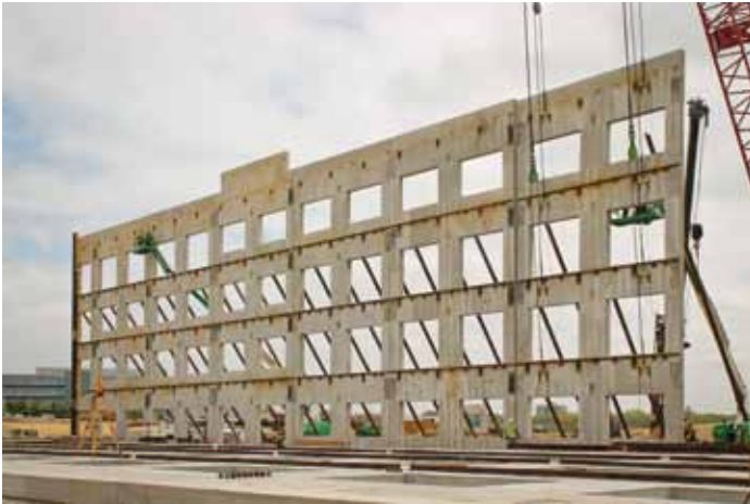
Erected panels from the building interior. Embedded plates at each panel joint will be connected for progressive collapse resistance.
