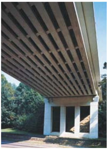
Underside view of Walnut Lane Memorial Bridge, showing the 13 post-tensioned concrete girders (1950).
