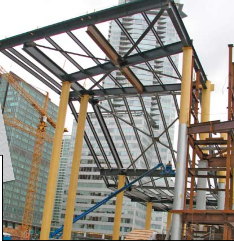
VCEC roof framing prior to roof deck installation showing supplementary diaphragm cross bracing.
