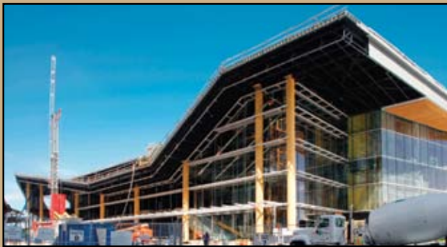
VCEC's 36-inch columns, sloped roofs with green roof systems and clear glazed perimeter walls.
