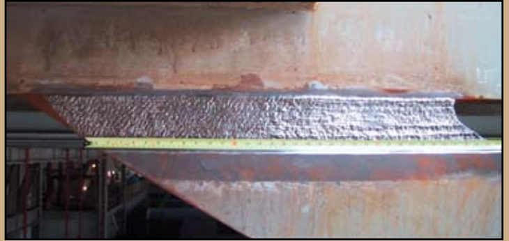
Field welding of key joints where assembled sections are limited by lifting capacity.
