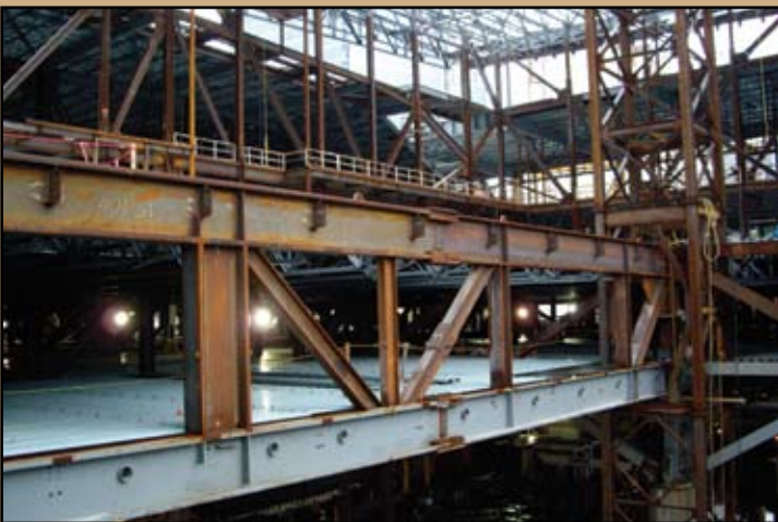
Parking Vierendeel trusses with drive aisle passing through trusses at 45-foot bay lines.
