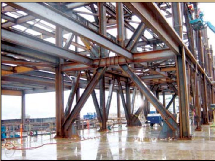
Eccentric braced bay seismic resisting system with bases cast into foundation slab.
