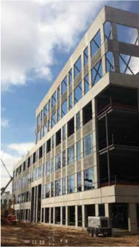
Erection of the upper panels on the east face as viewed from the northeast corner. Courtesy of Big 4 Steel Services, L.P.
