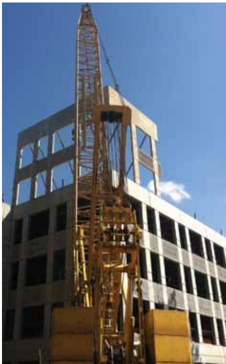
Erection of the upper panels on the northwest corner. Courtesy of Big 4 Steel Services, L.P.
