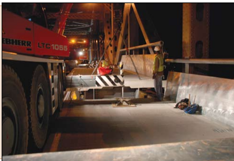
Installation of exterior precast deck panel, including permanent steel barrier, at main span, ready for vehicles to ride on in the morning.
