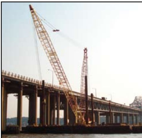
Barge-mounted crane is used to replace deck. Courtesy of New York State Thruway Authority.
