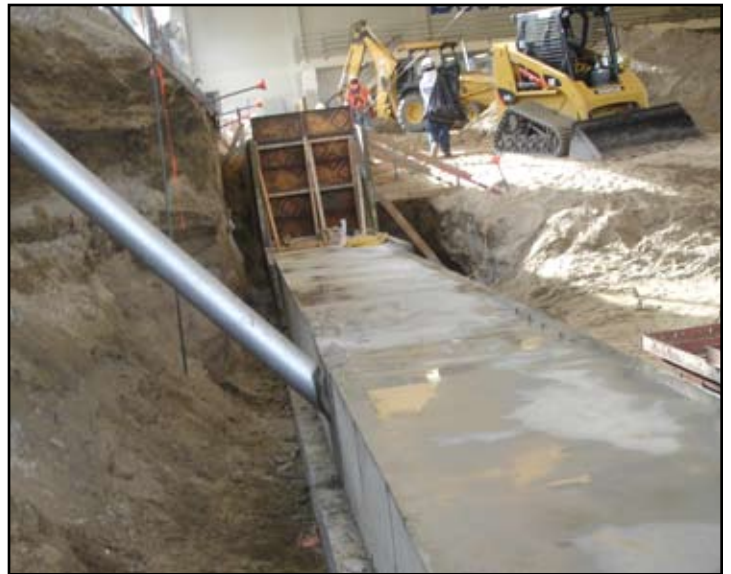
Figure 4: Footing poured, encasing base of shoring strut to be left in place.
