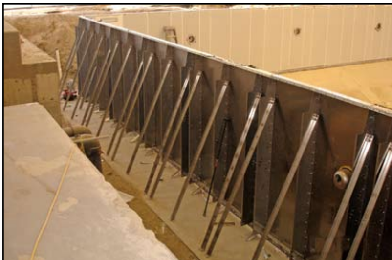
Figure 6: Stainless steel pool wall panels in place with partial supporting struts at deep end of pool.
